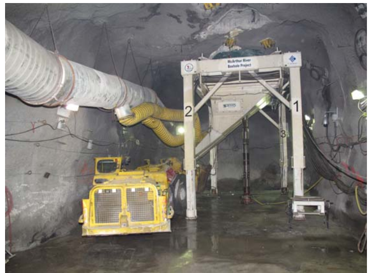
Figure 6 Muck chute, and extraction chamber set up (McArthur River Operation, 2010)
